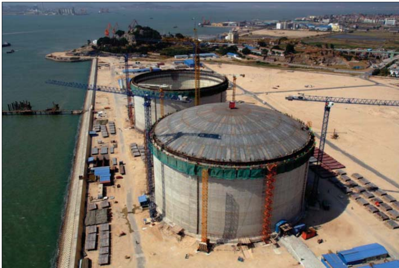
CB&I is building an LNG terminal in Xiuyu, Fujian Province, China, for CNOOC Fujian LNG Co. The terminal has Phase I capacity of 2.6 million tonnes/year with Phase II expansion under planning. The terminal is to begin operating in early 2008. Photo from CB&I.
