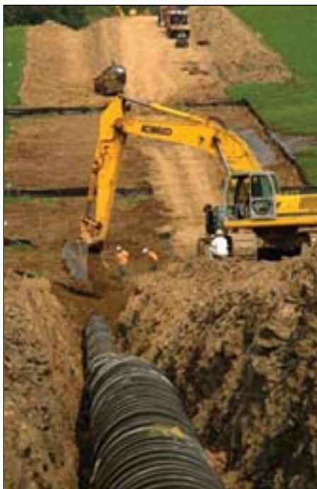
Construction includes 6 miles of 30-in. pipeline on the Northeast ConneXion-NY/NJ natural gas expansion project by Tennessee Gas Pipeline, subsidiary of El Paso Corp. Photo from El Paso.
